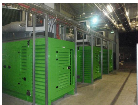
Fig. 4 A Combined Heat and Power (CHP) Station designed and installed by Aquafuel Research (UK) to deliver 1.5 MWe and 1 tonne/h steam powered by renewable biofuel
