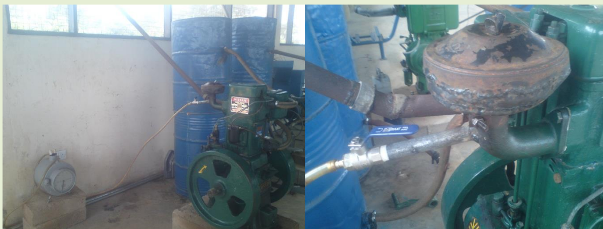
Fig. 2: Left: Section showing connections from the biogas pipeline through the gas meter into the converted dual-fuel engine.
