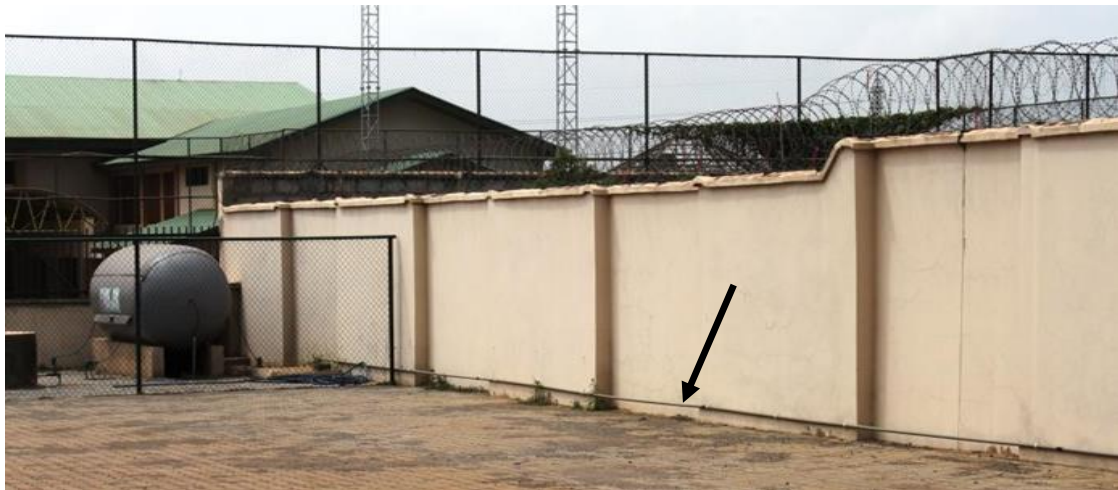
Figure 3: A picture showing a portion of the piping system (arrowed) used to transport the biogas to the school's kitchen and labs.
