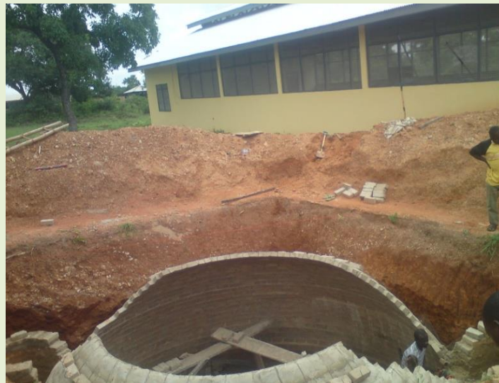
Fig. 1: An underground Anaerobic Digester located behind the Processing Hall.
